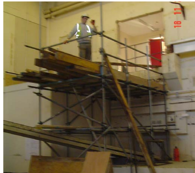
Build-up of shuttering for the TA3 bunker. The doorway hanging in mid-air is the door into Laser Area 3.
