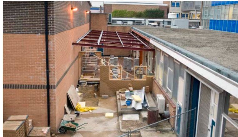
The Mechanical Workshop and Target Preparation Laboratory were refurbished in 2008, extending into a new corridor built between the old laboratories in R1 and the side of Vulcan TAP. (08EC1384)
