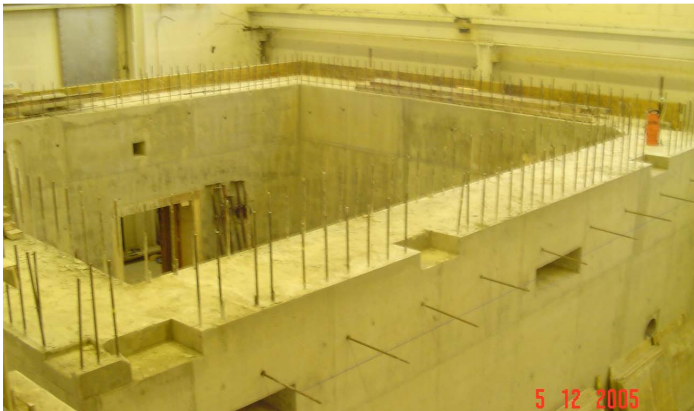
Target Area 3 bunker from the south east corner showing the metre-thick concrete walls, December 2005. The roof of TA3/floor of LA3 has yet to be added so you can see the entrance door to the bunker.
