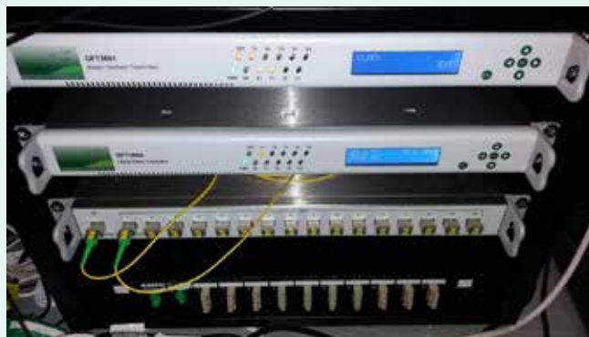
Installation of the Greenfield Master Oscillator and Slave Unit in the Front-End Oscillator Room.
