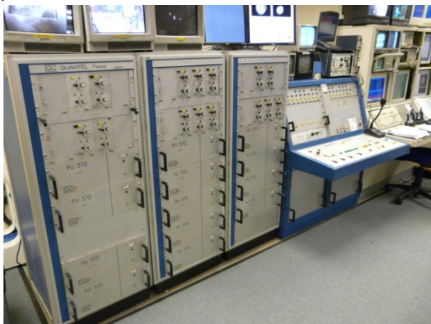
Figure 1 – Old Quantel units inside the Vulcan Main Control Room.
